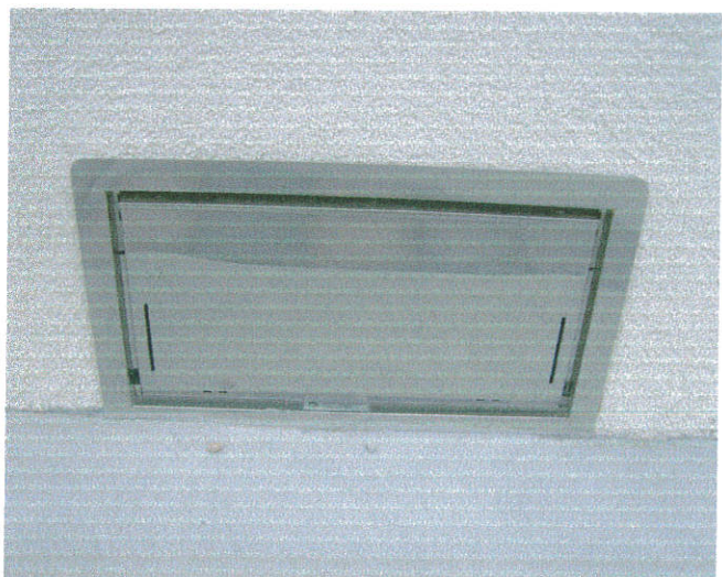
Smart Vent (4) in Garage Date Taken: 04/09/2008
